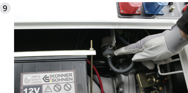
Air can get into the fuel system of the diesel generator, which can cause start-up complications. Therefore, if the generator does not start, you must perform the following steps: Look at the fuel filter, it may not be completely filled with fuel. Take the filter in your hand and try to remove air from it by changing its position (horizontally / vertically). Then try starting the generator again.
